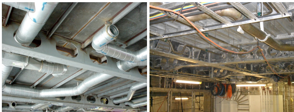
Figure 15: Typical 'tween deck depths for service runs (images courtesy of BMT Nigel Gee).
